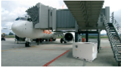
Piller ground support for passenger boarding bridge
