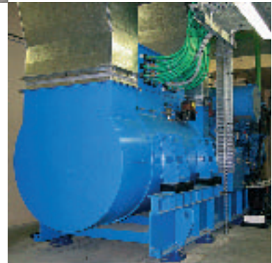
Diesel UNIBLOCK Dynamic UPS systems, Orly Airport, France
